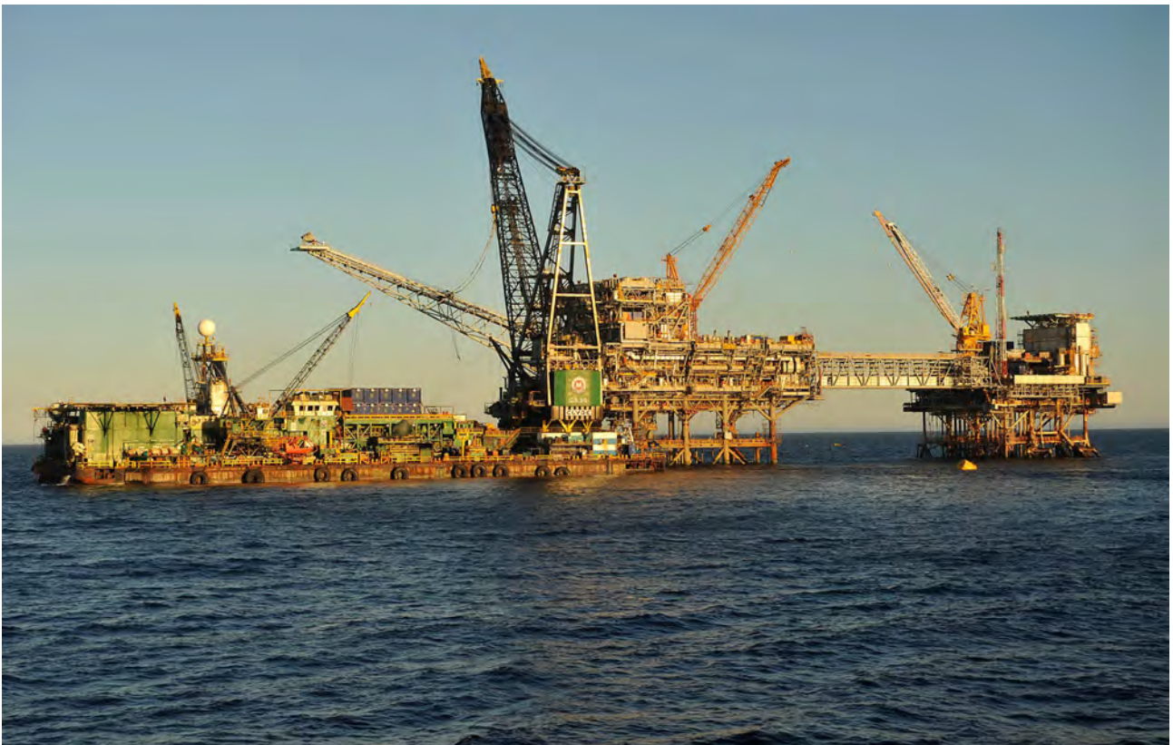
Figure 6 – Final positioning of the flare boom on the Marlin B platform using the derrick lay barge DB30 crane.
