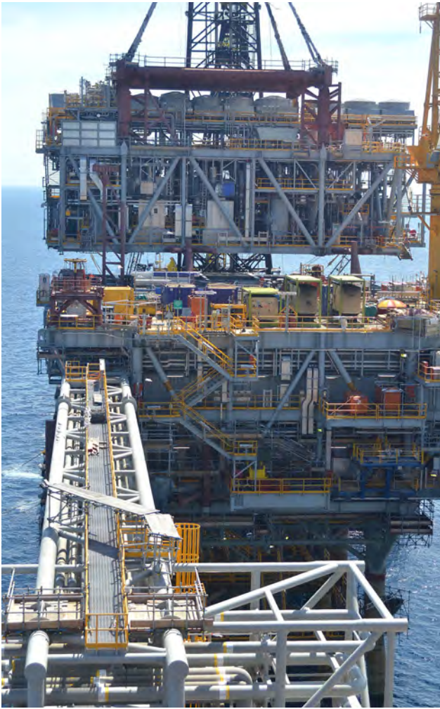
Figure 5 – Marlin B with 3 modules installed, and the final module being lifted into position by the derrick lay barge DB30.
