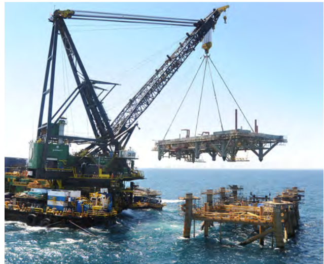
Figure 2 – Module Support Frame being lifted into position on the Marlin B jacket by the derrick lay barge DB30.
