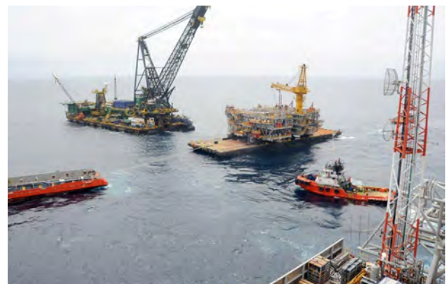
Figure 4 – Marlin B modules waiting on the equipment barge in front of derrick lay barge DB30.
