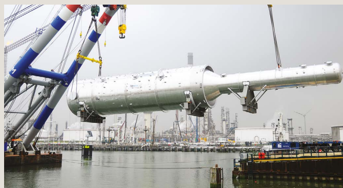
The vacuum fractionation tower, the largest piece of equipment to be placed on the foundation intact, arrives at ExxonMobil's Rotterdam, Netherlands, refinery in October 2016.
