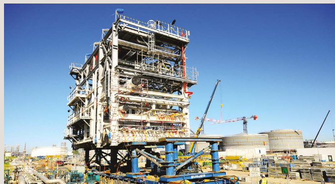
ExxonMobil engineers work to install the pre-assembled racks (PARs) at ExxonMobil's Rotterdam, Netherlands, refinery in June 2017; these are commonly referred to as the 'spine' of the hydrocracker.
